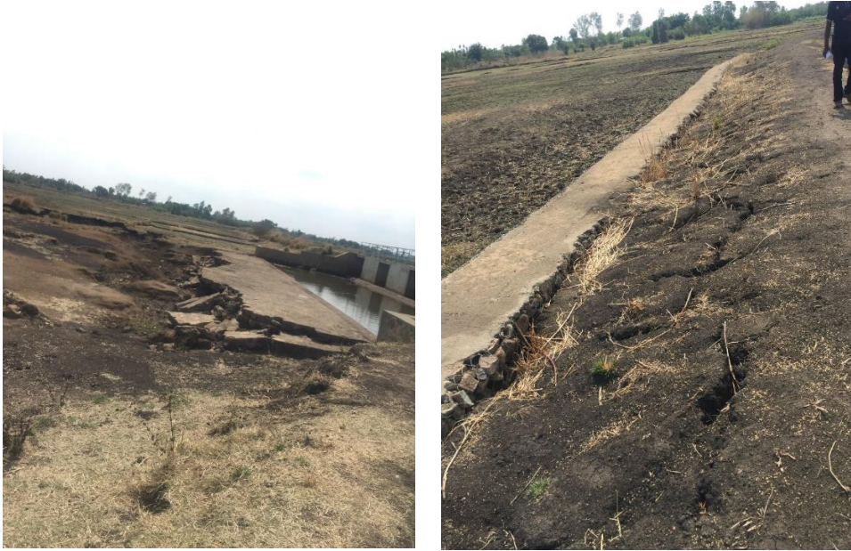
Figure 2 Intake at Naming'azi irrigation Scheme
