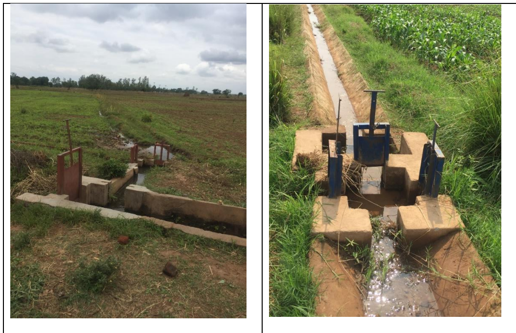
Figure 5 Fully functional Hydraulic Structures Timoti Irrigation scheme
