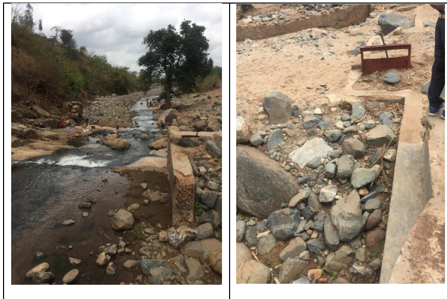
Figure 3 Damaged intake headworks at Masenjere Irrigation scheme.
