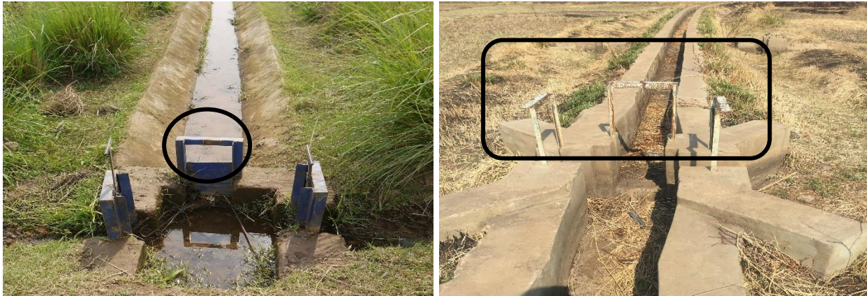
Figure 4 Hydraulic structures with gate components missing.
