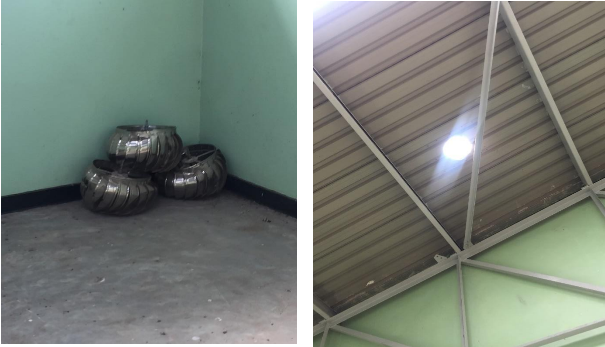
Figure 2 Roof Air vents not installed at Mphinga VAC
