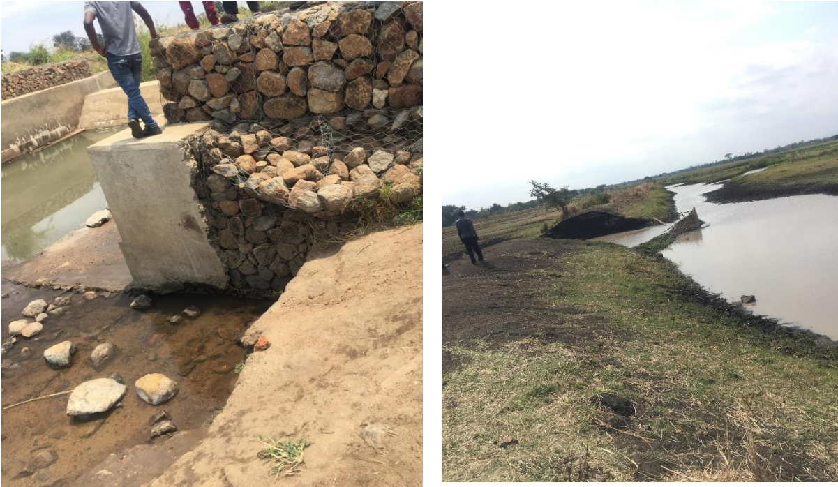
Figure 1 Rock gabions at Zumula A irrigation scheme and the damaged Dyke at Naming’azi Irrigation scheme in Machinga.
