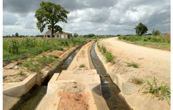
Canals, access road, toilets and resting shed at Njage irrigation scheme, Mlimba
