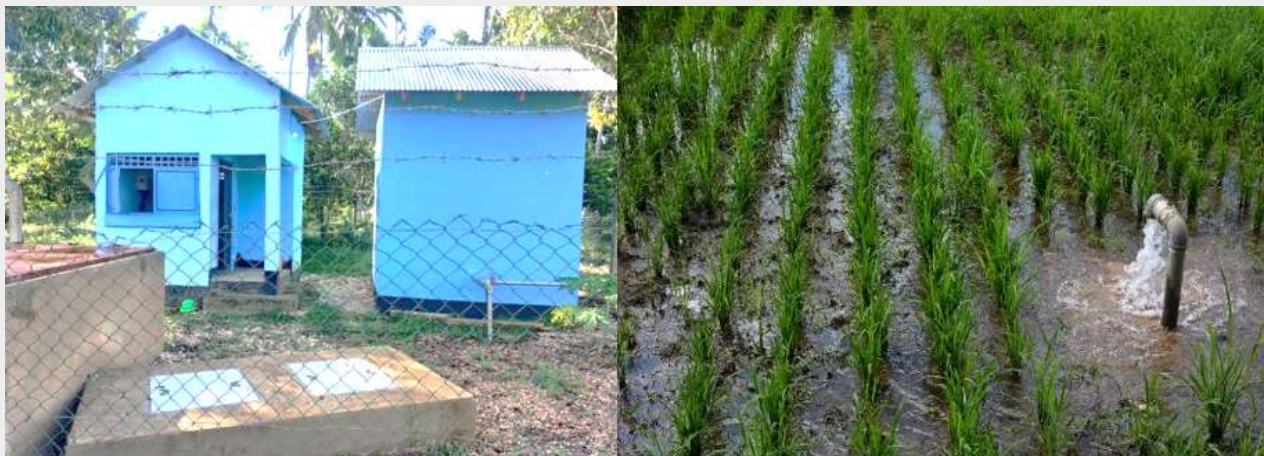
Pumping unit (left), individual plot (right) equipped with hydrant for watering at Koani scheme in Zanzibar (Source: Annual Reports)
